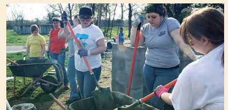
L-R, Alicia Vargas, Kara Wheaton and Katie Armagost mix concrete to be used while building the block foundations of a Habitat for Humanity house.
